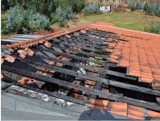
Figure 3: Roof damaged during the fire in Funchal (Portugal) in 2016 [7]
