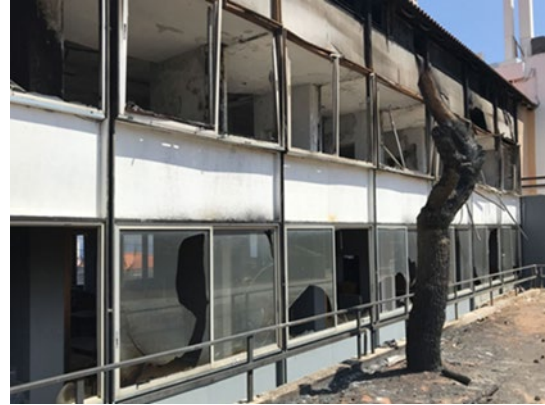
Figure 4: Broken windows in Neos Voutzas-Mati (Greece, 2018) due to the combustion of a pine tree [7]
